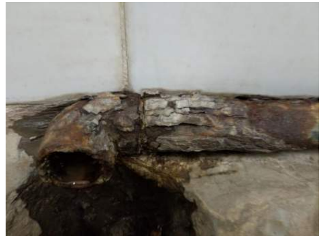
Fig. 3. Photograph of corroded GI pipe line of raw water at Kirandul, Bailadila Iron ore Mine, India.
