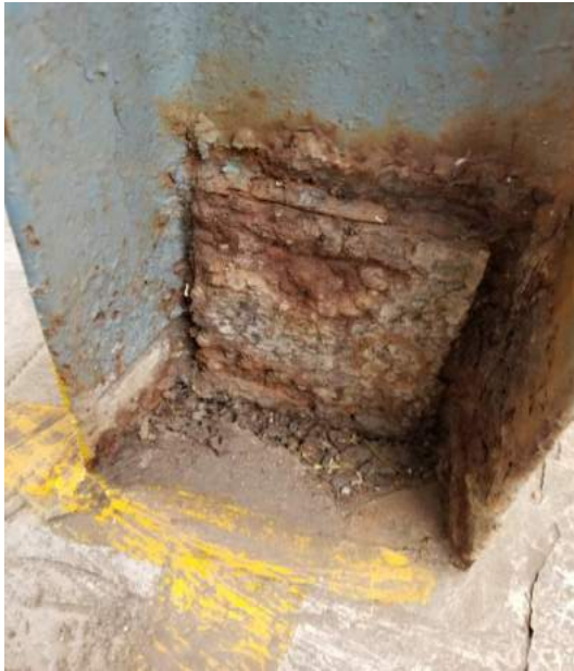
Fig.4 Photograph of corroded process plant structural support at Kirandul, Bailadila Iron Ore Mine, India
