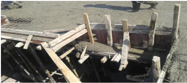
Fig 4: Wastages of Concrete ( Source: Veda Construction)
